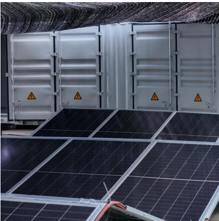
Folding solar system power generation cabin
