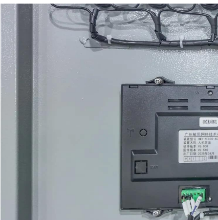
Solar Container , Large Mobile Solar Power ...
