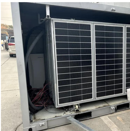
10kW Growatt Grid-Tie Inverter
