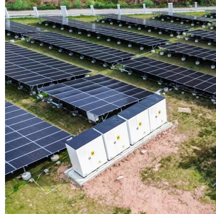
Solar Container , Large Mobile Solar Power ...
