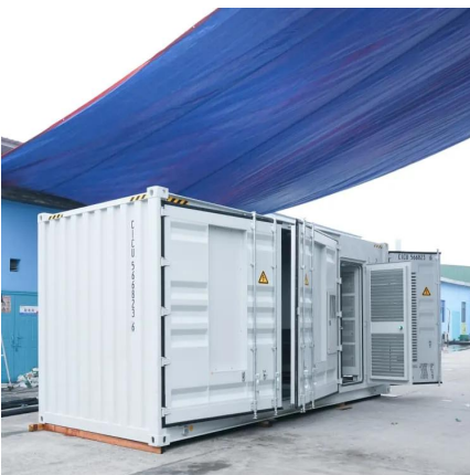
Masdar's first battery storage project in the UK begins ...
