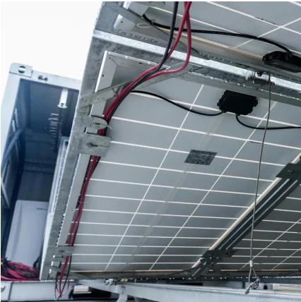
containerized battery storage, SUNTON POWER
