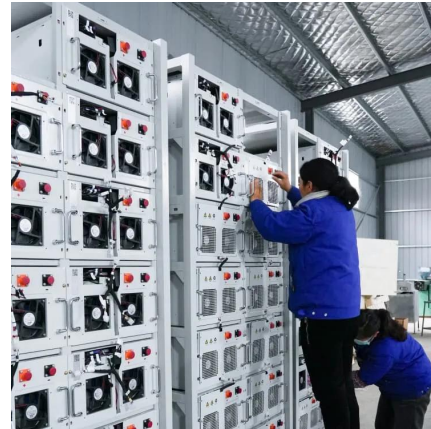
2MWH Container Solar Battery Storage ...
