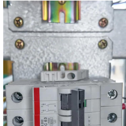
SUNWAY 30KW 51.2KWH Energy Storage System
