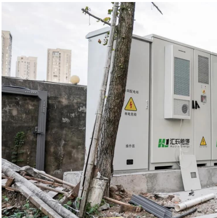
Lithium Battery Container
