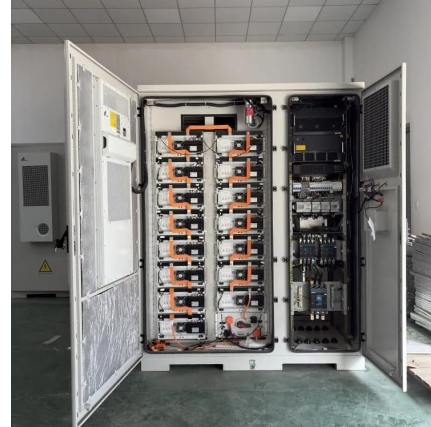
600KW 1.26MWh ESS Battery Storage Container
