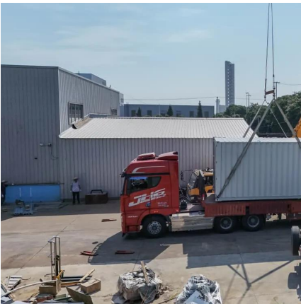
600kw 40ft Containerized Energy Storage Solution 2MWh...
