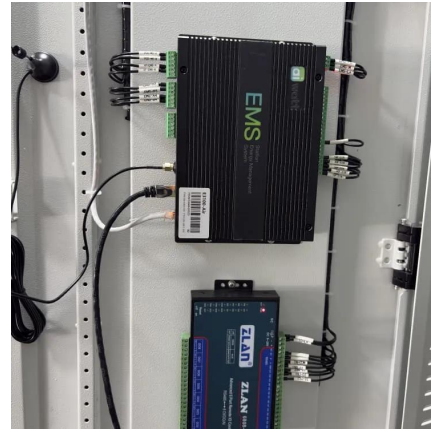
60kw Micro-Grid Solar Power System with Lithium Storage
