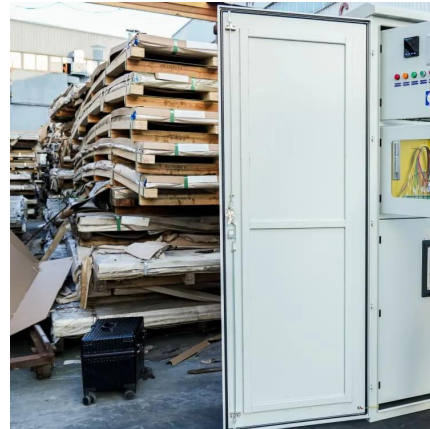
40FT Container Battery Storage 800kw off ...
