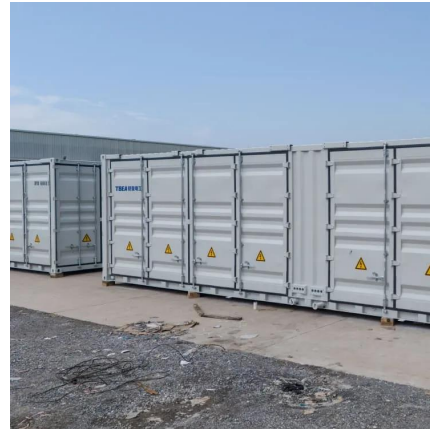
20kW Solar Package - B& K Solar
