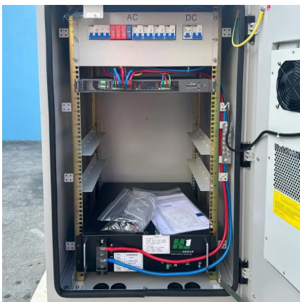
Andorra city energy storage battery enterprise
