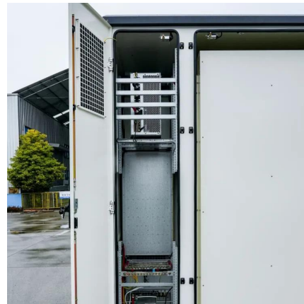
Understanding Battery Energy Storage ...
