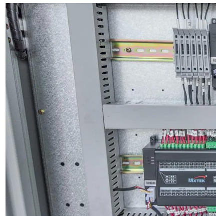
200kw Solar Monocrystal Power Industrial Container Storage
