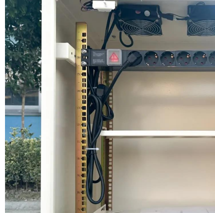
Cabinet Energy Storage System , VREMT
