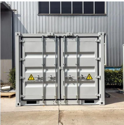
The Barbados Battery Energy Storage Systems ...
