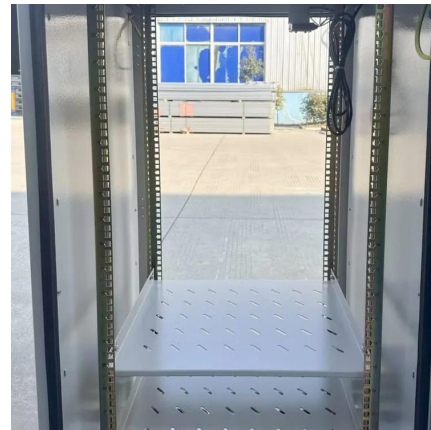
The Barbados Battery Energy Storage Systems (BESS) ...
