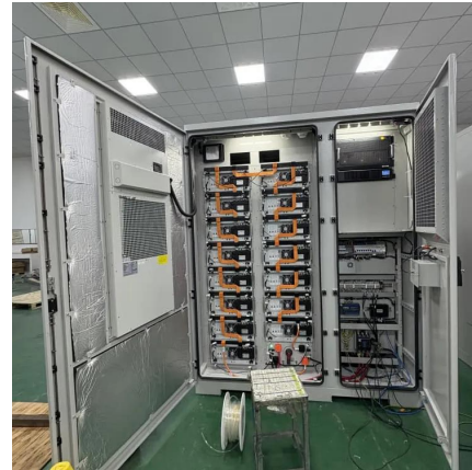
BESS 1MW 3.2MWh AC 480V Three Phase ...
