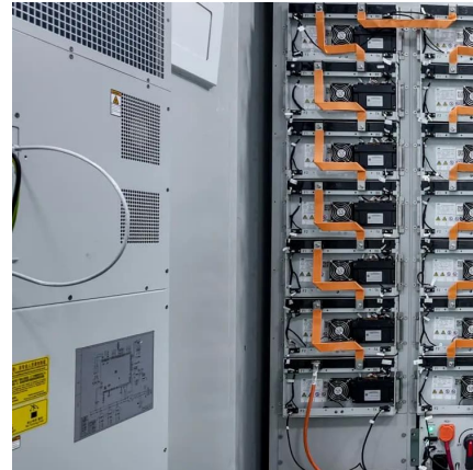
Energy storage container, BESS container
