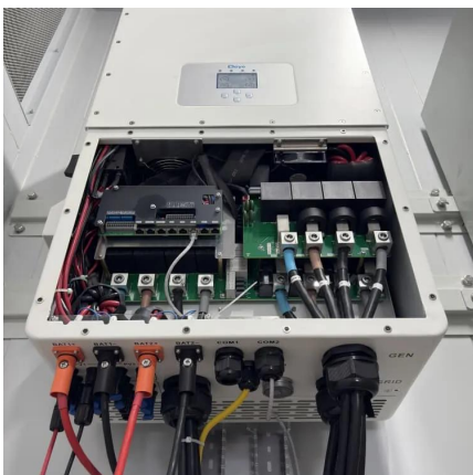
Battery Energy Storage Container: Differences and ...
