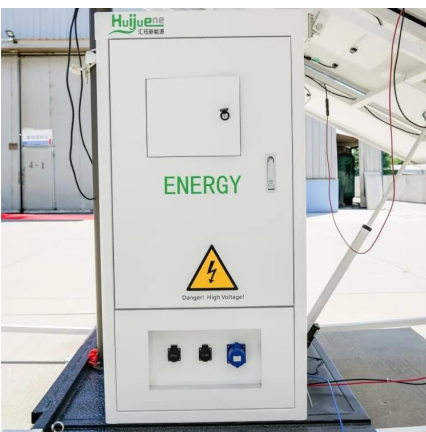
Containerized Battery Energy Storage Systems (BESS)
