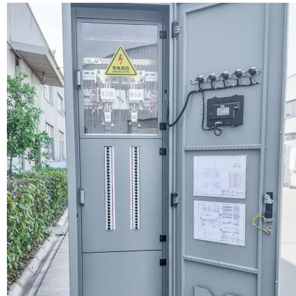
LLVD & BLVD in Base Station Power Cabinets
