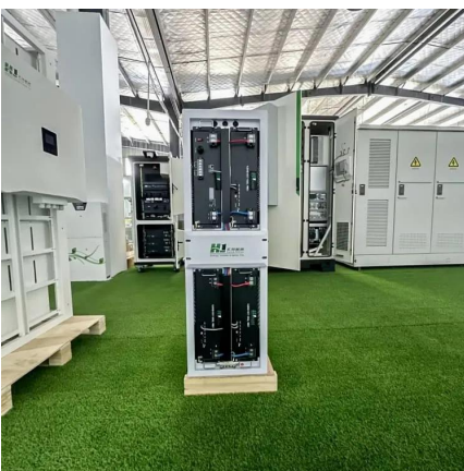
Energy storage container, BESS container
