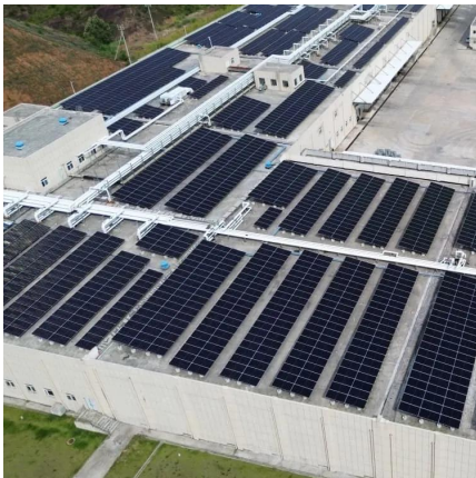
Brazil 500kw solar power plant
