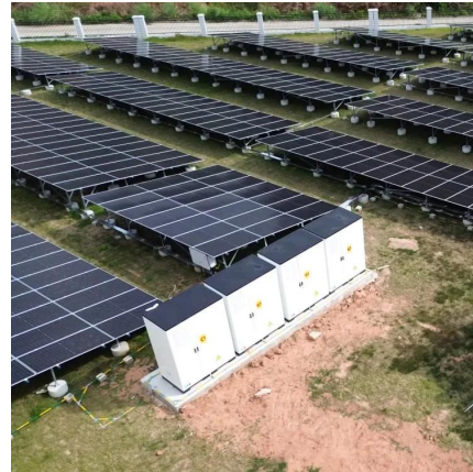
1MW/2MWh Energy Storage Container System
