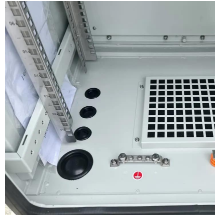
200kw industrial commercial hybrid solar system battery ...
