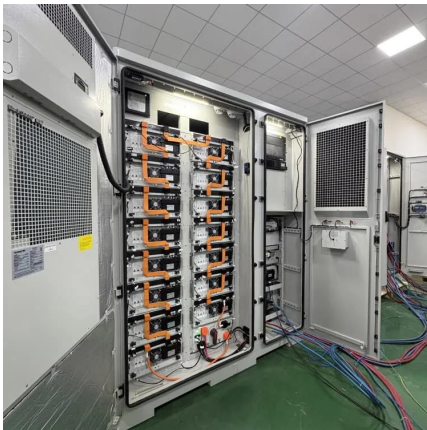
Energy storage container, BESS container
