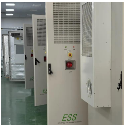
Jinko Power, EnergyStorage
