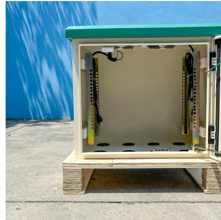
Sterling & Wilson Completes Greenfield Data ...
