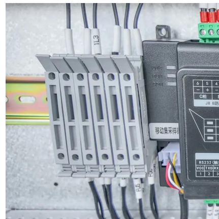
Telecom Base Station Battery
