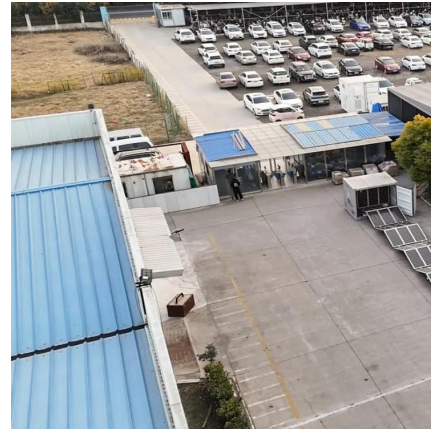
Overview of Telecom Base Station Batteries
