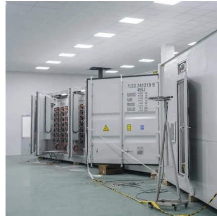
PWD Grid-Connected and Off-Grid Switching Cabinet System
