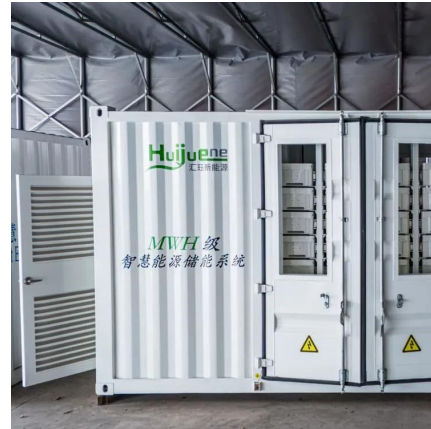
The power system for an outdoor hybrid ...
