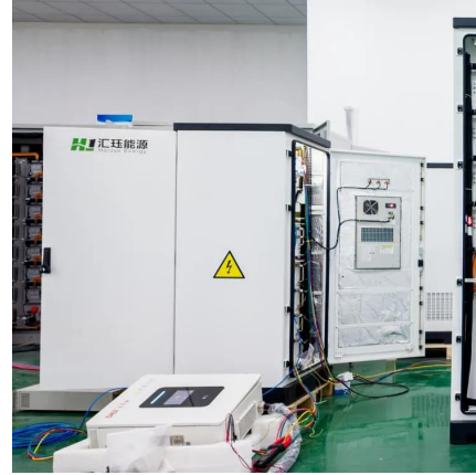
Cabinet Energy Storage System , VREMT
