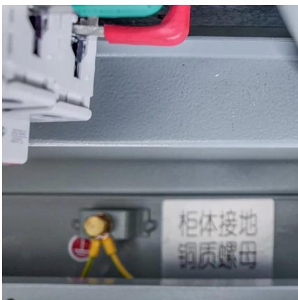
Guinea Bissau Container Battery Storage Cabinet
