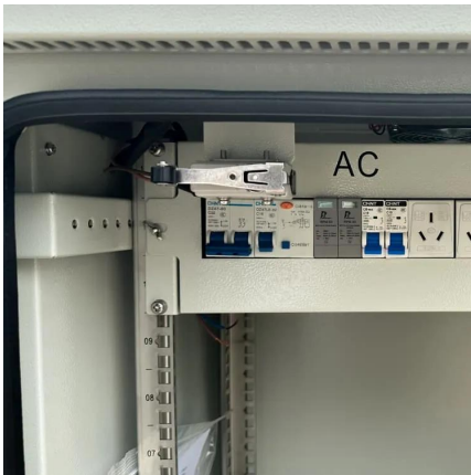
Solarcontainer: The mobile solar system
