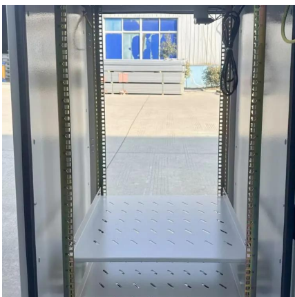
Outdoor Communication Cabinets and Power...
