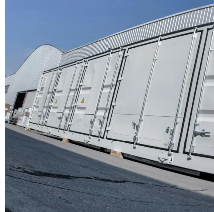
Emergency Power Container for Disaster ...
