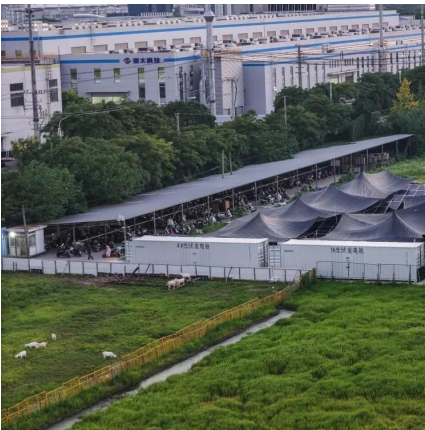
Energy Storage Solution (ESS) , HUAWEI...
