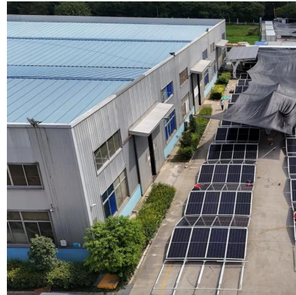
Energy Storage Equipment, Energy storage solutions,...
