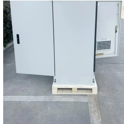
Cambodia's First Grid-Forming ESS by Huawei & SchneiTec
