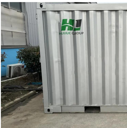
HUAWAI BATTERY STORAGE SYSTEM POWERING A...
