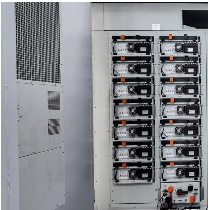
Huawei Saint Lucia pack batteries
