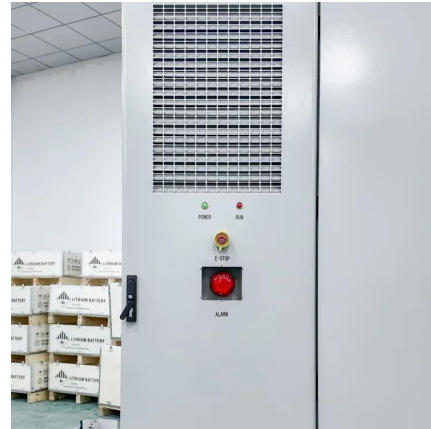
Solarcontainer: The mobile solar system
