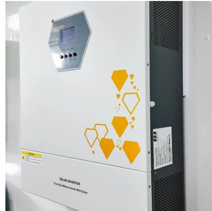
Solar Panels & Installation in Iraq , Baghdad, ...
