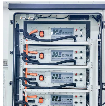
NPC , Solar , Roof top mounted 30kVA, 3Ph with 30KWh Energy Storage
