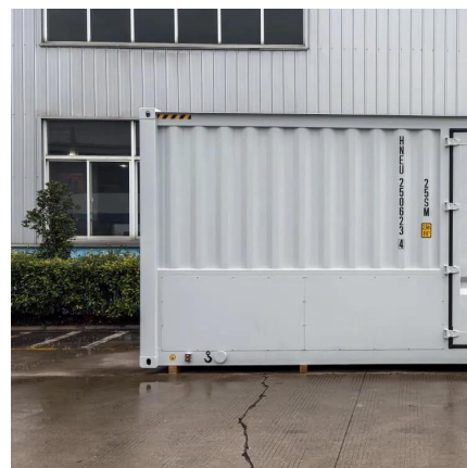
Battery Storage , RWE in Ireland
