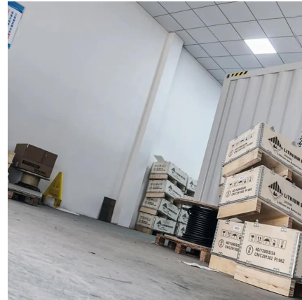
Fire breaks out at German lithium battery storage station
