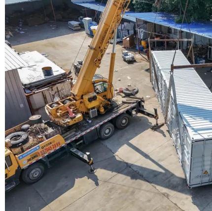
containerized battery storage , SUNTON POWER
