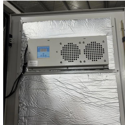
Energy storage container, BESS container
