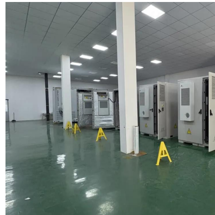
Lithium Battery Energy Storage Cabinet
