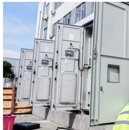
Madagascar Solar Air Conditioning Plant A Sustainable ...
