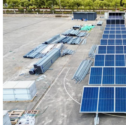
Manama photovoltaic energy storage project
