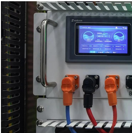
Outdoor communication cabinet
