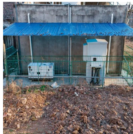
Nicosia 5g base station equipped with energy storage
