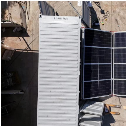
5G Base Station Solar Photovoltaic Energy ...
