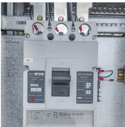
NICOSIA POLY NEW SOLAR CONTAINER POWER STATION
