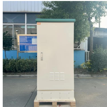
NICOSIA ENERGY STORAGE CONTAINER , Solar Power ...
