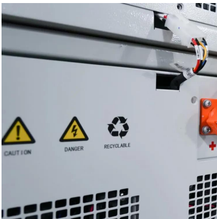
100kW Off Grid solar system (115.2kWh)
