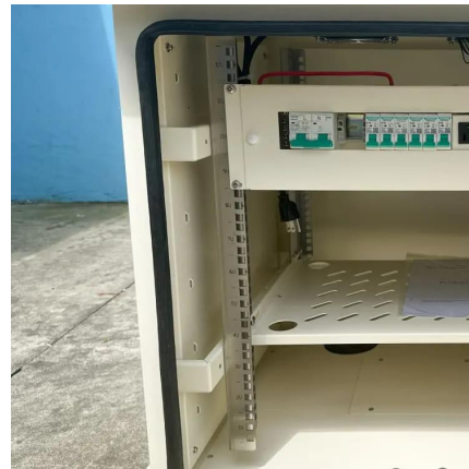
NOUAKCHOTT COMMUNICATION ENERGY STORAGE BATTERY
