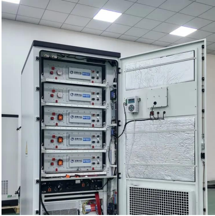
EK-SG-R01 Communication container station
