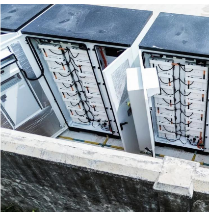
NUKU ALOFA WIND SOLAR AND ENERGY STORAGE NEW ENERGY ...
