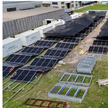
THE NUKU'ALOFO ENERGY STORAGE PLANT FACTORY POWERING
