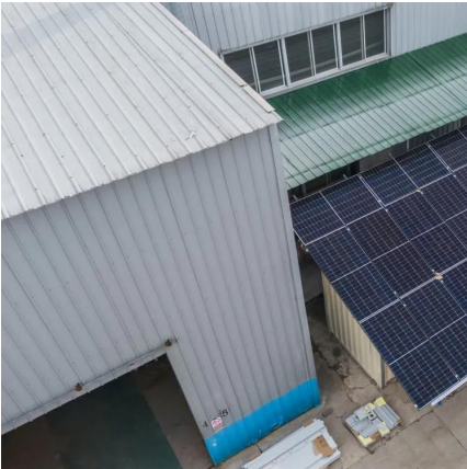
Vietnam grid-tie 5kw solar system
